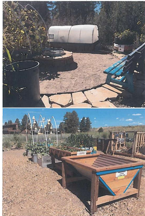
Above: Wheelchair path prior to final compaction with flagstone edging. Below: Constructed beds on July 13, 2019. (Jan Busco, MNA)
