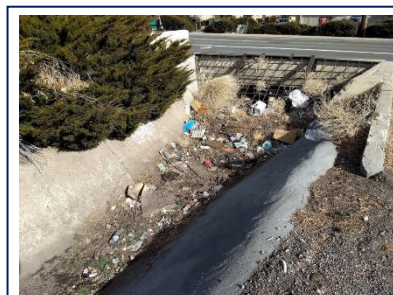
Debris clogs the grate in Fanning Wash (before).
